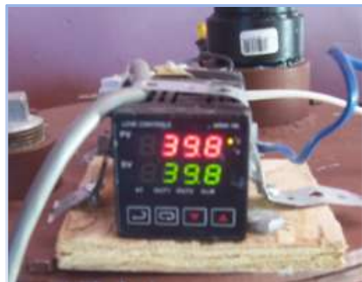
Figure 1.2.3. Control temperature system
