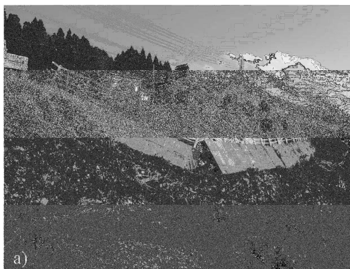
Figure 2.15 Damage of retaining wall along National Highway Route 17
