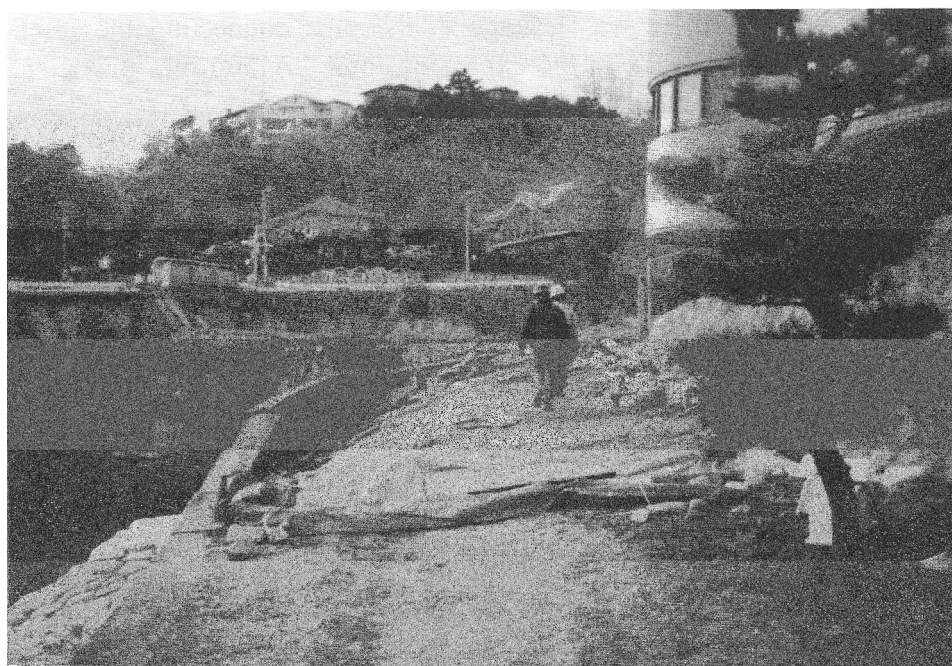
Figure 2.9 Cracked retaining wall (left) at Motoyama water purification plant intake box
