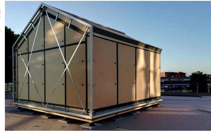
Figure 201 / Installation of the holed galvanized folded steel sheet and of aluminium profiles - On-site - University Campus, Catania (CT)
