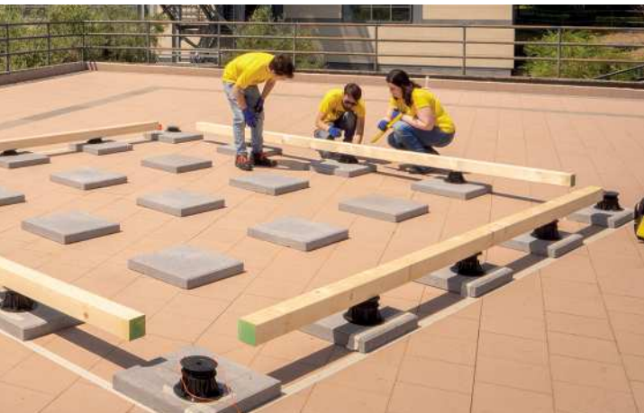
Figure 185/ Adjustment of supports and fixing of wooden beams - On-site - University Campus, Catania (CT)
