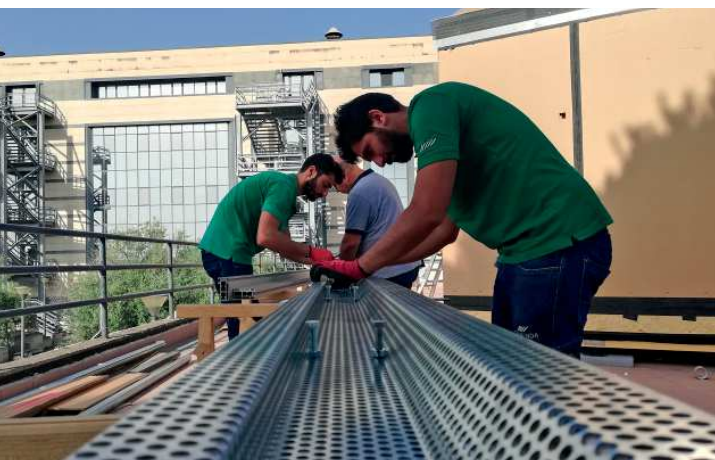
Figure 200 / Preparation of the holed galvanized folded steel sheet - On-site - University Campus, Catania (CT)
