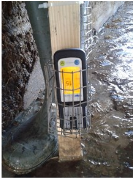
Fig.22 - Ammonia concentration measurement with the portable instruments placed in the wooden facility, before the treatment.
