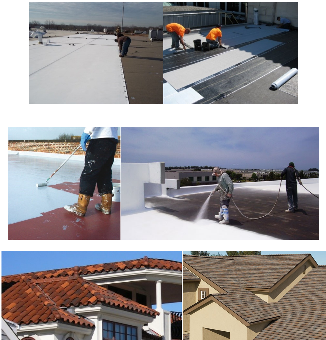
FIGURE 3.2: Typical cool roofs solutions: single ply membranes and modified bitumen in the first row, coatings in the second row and tiles and shingles in the last row [Internet]
